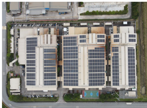
Figure 4 Picture of solar power installation of SAT-2 Plant with installed capacity of 1.5 MW
